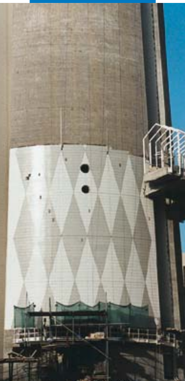
An example of an installation of klinker on concrete with Kerabond + Isolastic - New Telecommunication Tower - Kuwait City (Kuwait)
